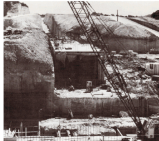
LAMPF construction is now underway. In foreground is the injector building foundation at the west end of the half-mile long beam channel.
